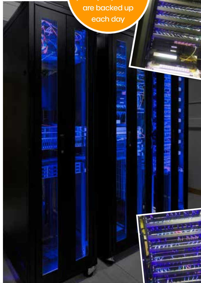
Skypark's state-of-the-art server room
